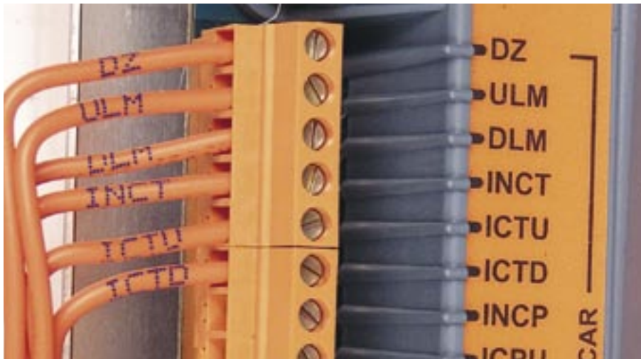
Typical label stamping at controller end
